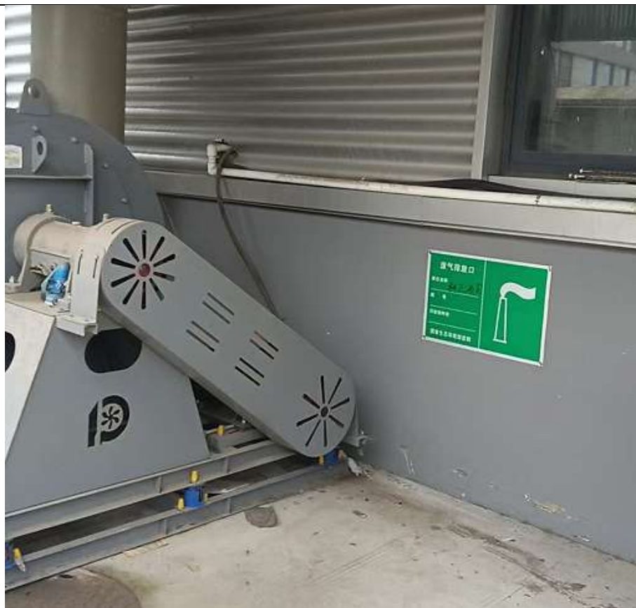
废气排放口标牌
